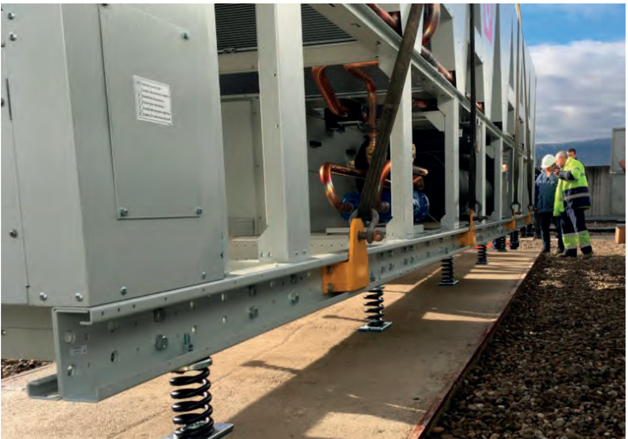
Ventilation system insulated with VIBRABSORBER
